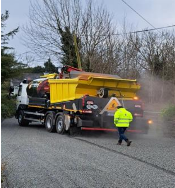
COMBI UNIT IN OPERATION AT SHANCLOUGH, KINVARA
