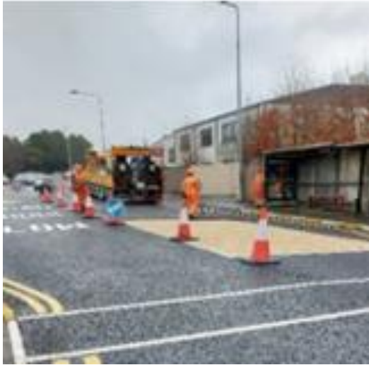
ANTI SKID SURFACE WAS INSTALLED AT THE PEDESTRIAN CROSSING ON THE FRANK STOCKWELL ROAD
